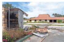
Much of the Jerome Golden Center building in West Palm Beach will have to be demolished, according to its new owners. GREG LOVETT/PALM BEACH POST
